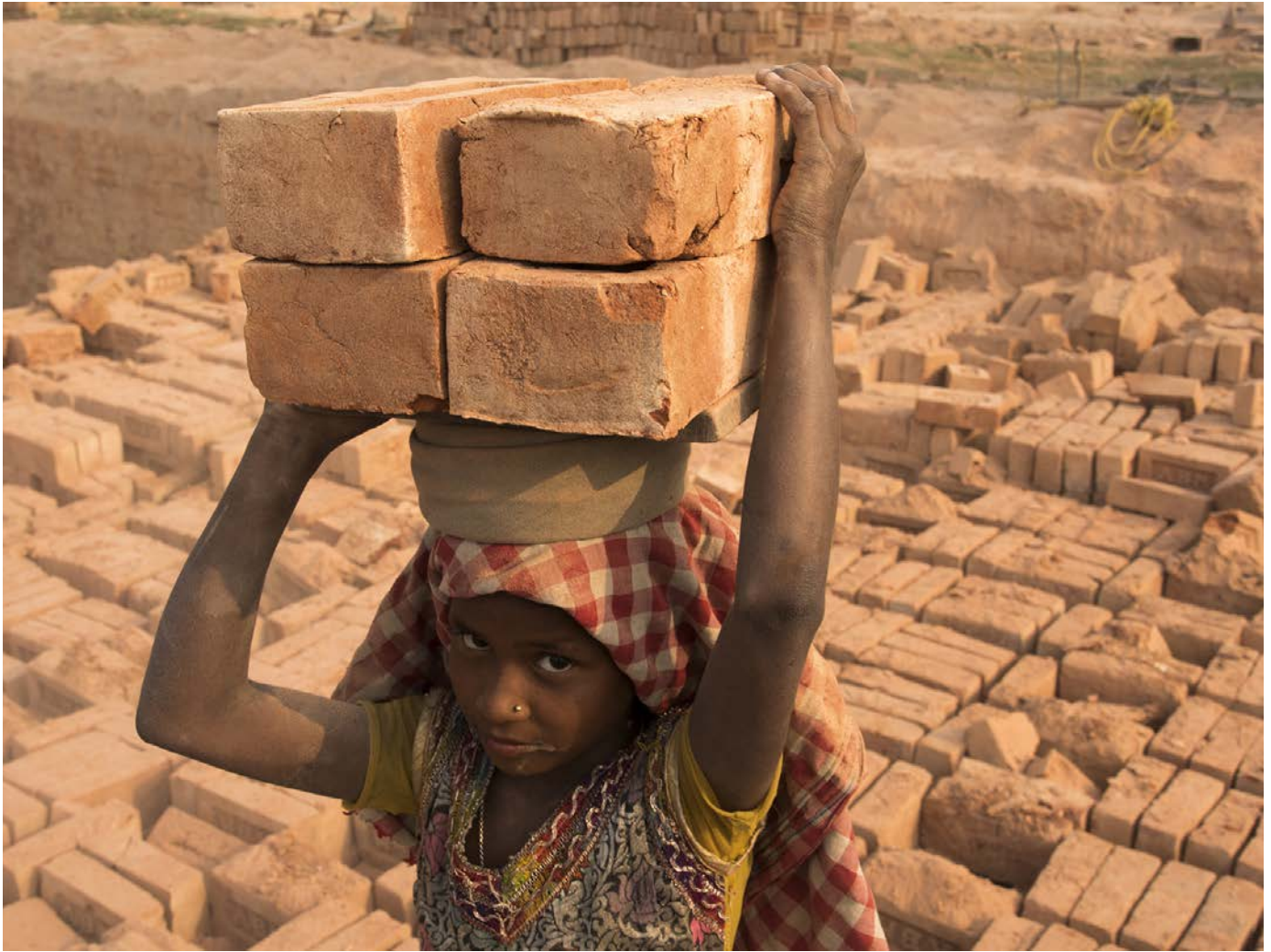
A child carries bricks on her head as a part of her daily job in West Bengal, India. Thousands of migrants from Bihar and Jharkhand work as unskilled labourers in the brick fields of West Bengal.
