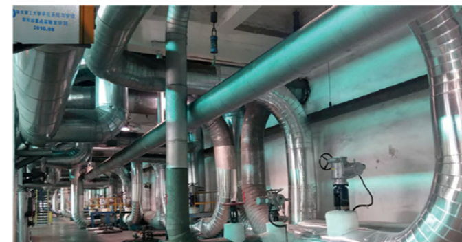
Technologies developed by ECUST researchers are applied in a monitoring and diagnostic system for high temperature and high pressure main steam pipeline.
