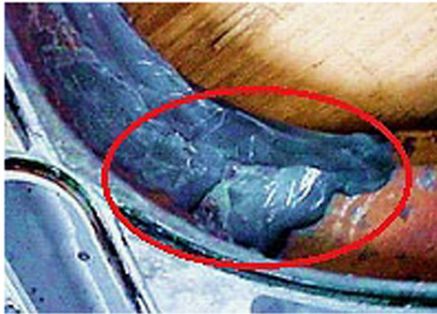
Figure 1. Failure caused by sand impact erosion of the mild steel.
