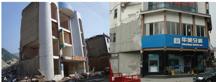
Fig. 2 The view shows the collapsed local hospital (A) and damaged local dental clinic (B) in the earthquake-hit Dujiangyan city
