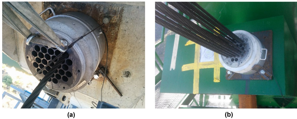
Figure 13. Tajo Bridge load cells: (a) load cell installation on cable-stayed pile; (b) load cell installation on cable-stayed tower.
