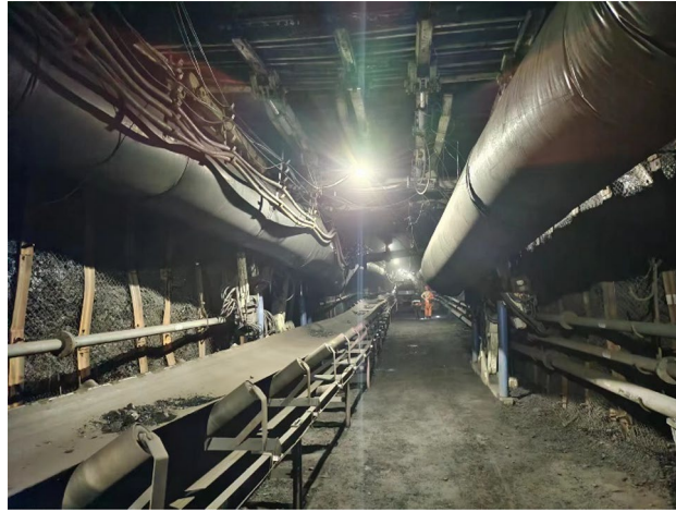
Figure 1. Real scene of the experimental tunnel.
