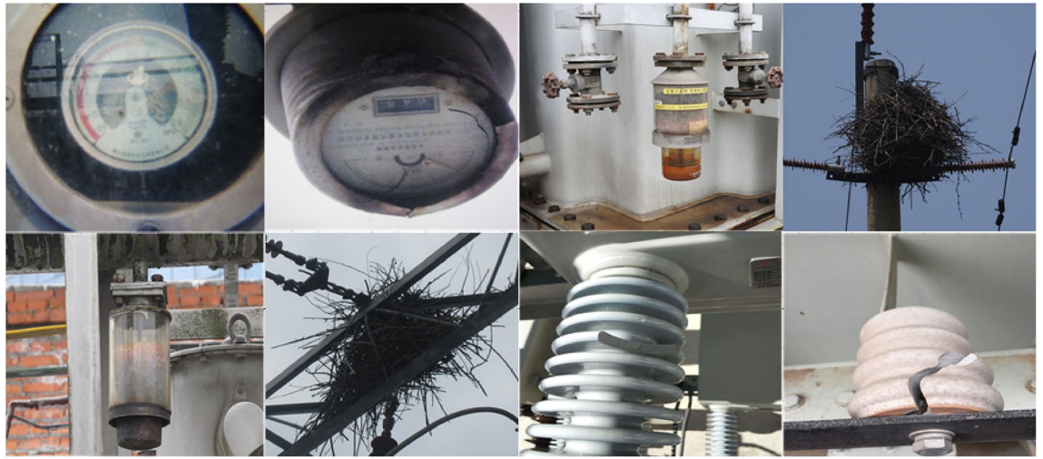
Figure 3. The dataset obtained by UAV from substation.
