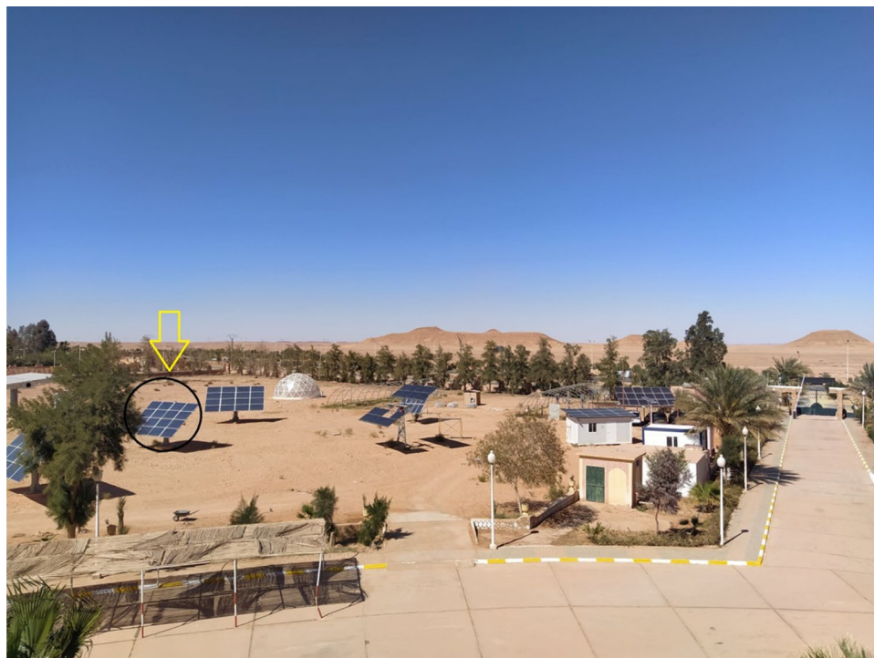
Figure 13. A photo of the investigated PV array.
