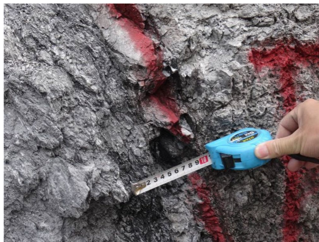
Figure 4. Rock cracks during slope excavation.
