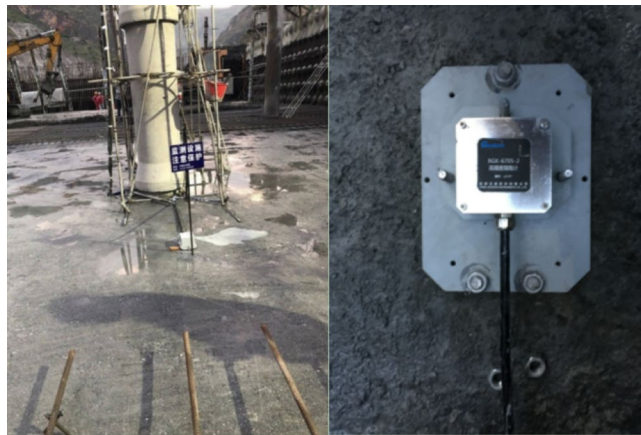
Figure 5. Displacement monitoring device.
