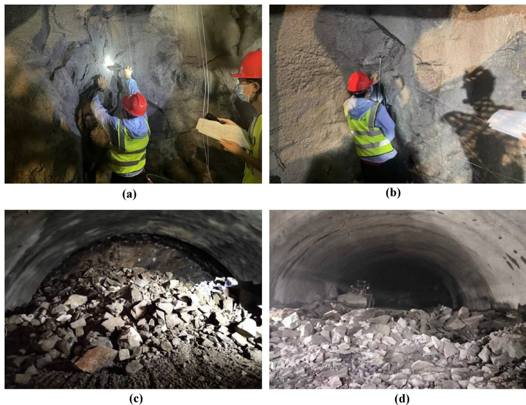
Figure 19. Blasting statistics of Lushan tunnel site. (a) Inspection and blasting program 1. (b) Inspection and blasting program 2. (c) Post-blasting debris 1. (d) Post-blasting debris 2.
