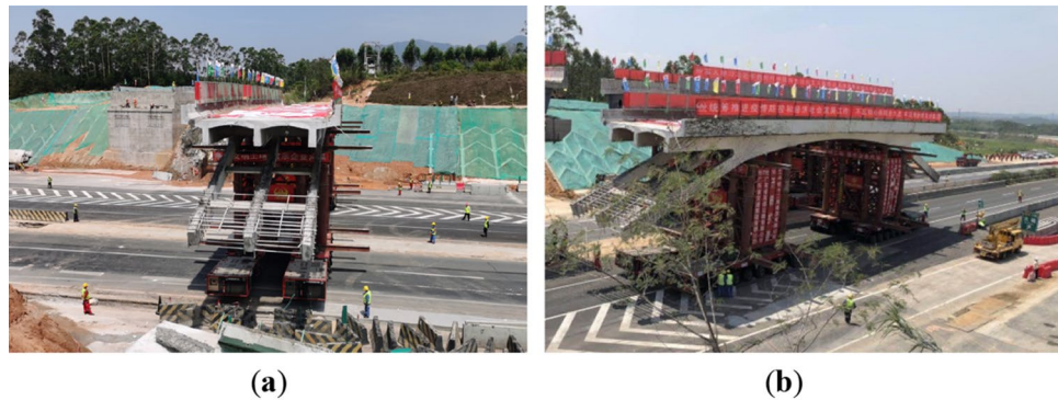
Figure 17. Movement of the cut bridge body (a) transversely movement (b) longitudinal movement.
