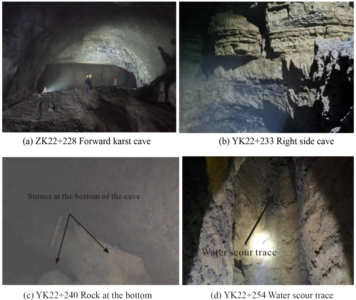
Figure 9. Karst cave in tunnel.
