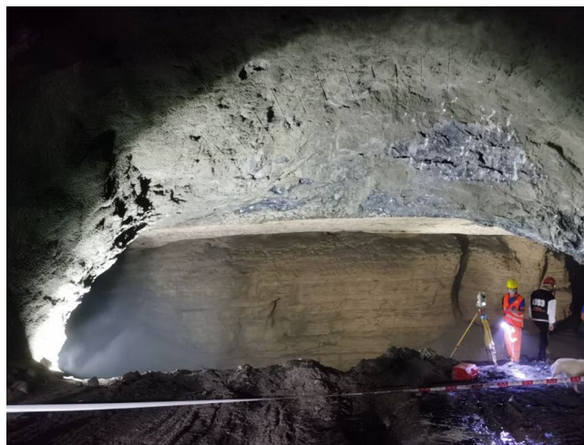
Figure 6. Tunnel face encounters karst cave.
