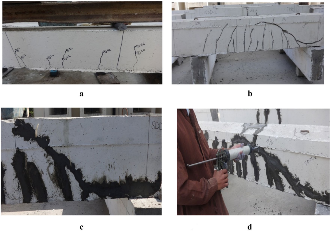
Figure 6. (a) Crack marking with respective load. (b) cleaning cracks and preparing for fill. (c) Sealing of cracks with PMM paste. (d) Injection of PMM into cracks.
