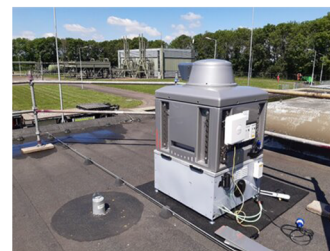
(c) Sensor setting on the cooling unit installed on the roof of the facility control room.
