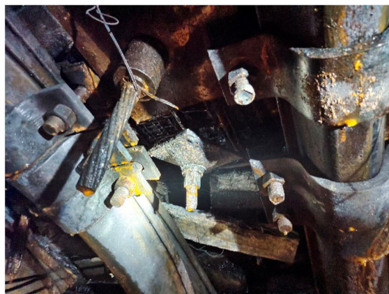
(a) Anchor failure
