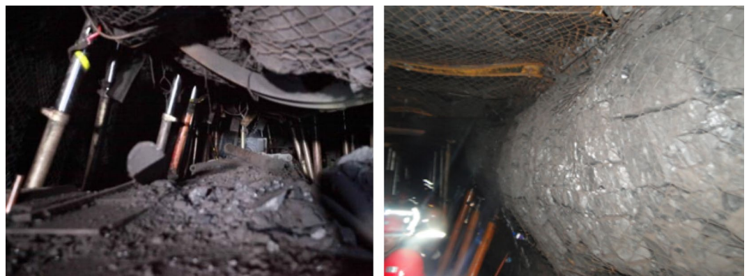
Figure 16. Excessive unloading pressure leads to serious deformation and damage to the roadway site.
