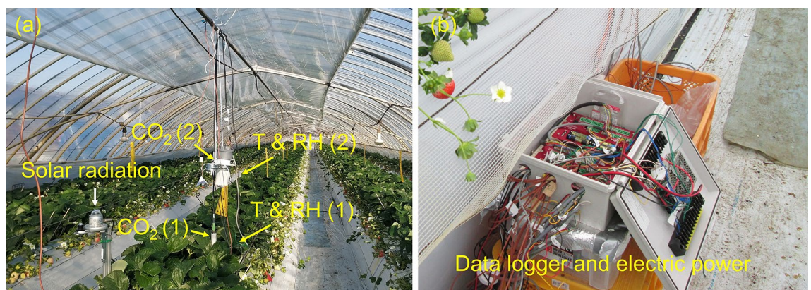
Figure 3. Photographs of the installation of the sensors at the Long Greenhouse centre (a) and the data acquisition system (b). The sensors included solar radiation sensors, CO 2 sensors (No. 1 and 2) and temperature and relative humidity (T & RH) sensors (No. 1 and 2).
