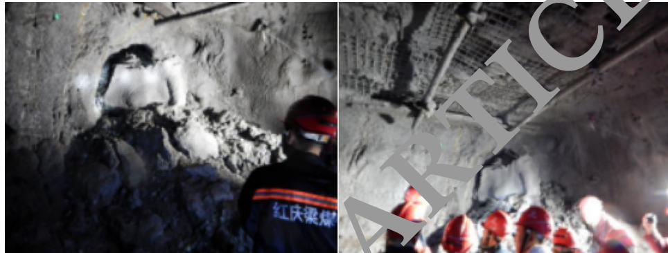
Figure 12. Collapse of site roofing.
