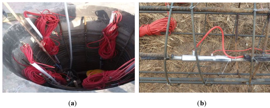
Figure 7. Site photograph of the sensor arrangement: (a) Pile top steel stress gauge wire layout. (b) Coaxial lap welding photo.
