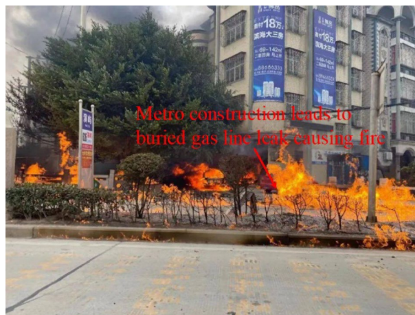
Figure 2. Gas pipe leak causes fire.
