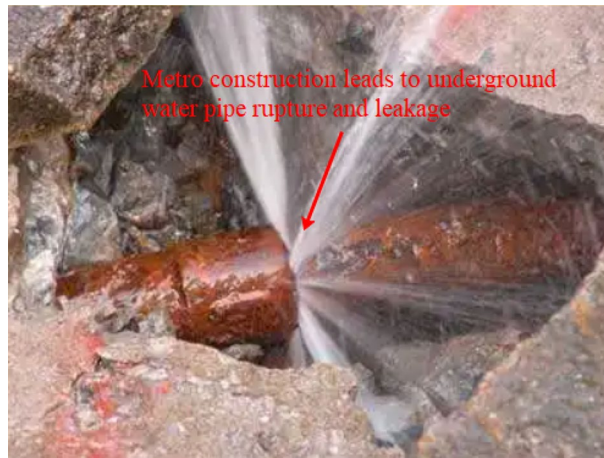
Figure 1. Rupture of water supply pipe due to metro construction.
