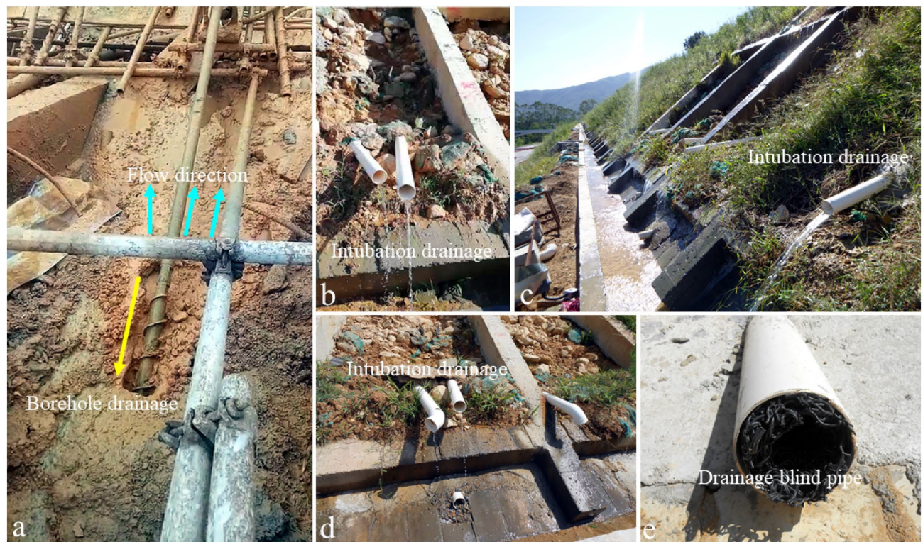
Figure 12. Drainage measures were taken to reduce landslide risk. (a) Borehole drainage (construction of deep horizontal drain hole); (b–d) slope insert tilted drainpipe; (e) buried drainage blind pipe.
