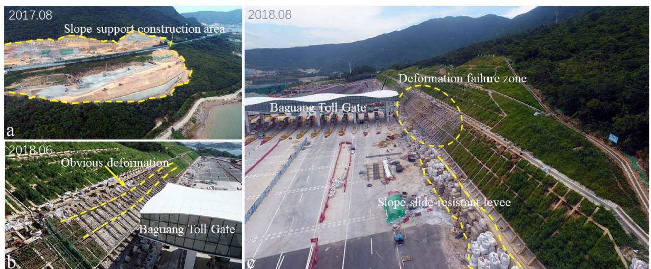
Figure 2. Typical stages before the formation of the Baguang Toll Landslide: (a) excavation of the Baguang toll station slope in the initial construction stage; (b) large deformation threatening the toll station safety; (c) slope supporting structure appears obvious deformation and failure area for suffering typhoon.
