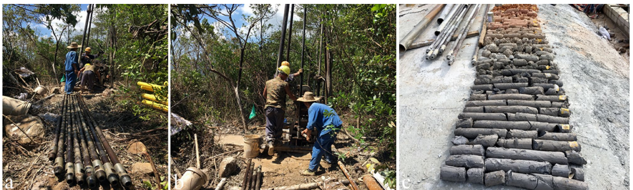
Figure 5. Drilling detection construction processes: (a,b) Drilling process and drill pipe installation; (c) complete core sample taken from borehole.
