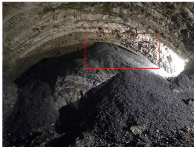
Figure 6. Collapse of the excavated face (DK80 + 407).
