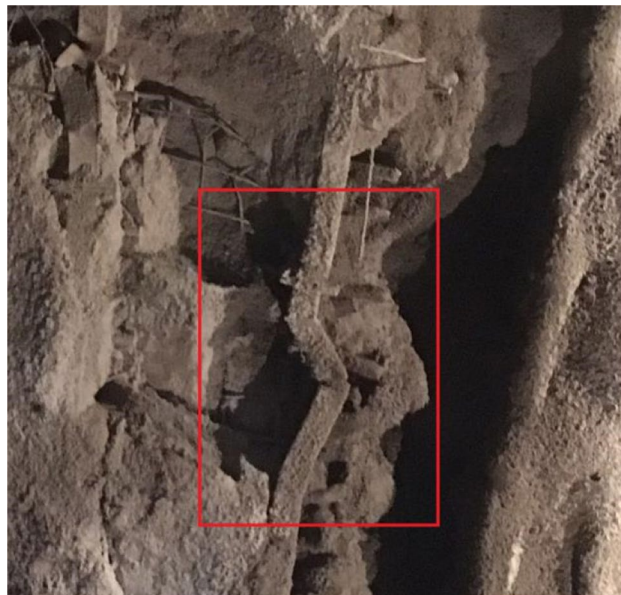
Figure 7. The failure of the steel arch frame at DK80 + 427.
