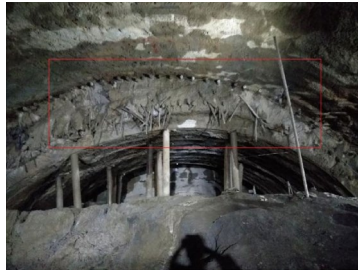
(b) The intrusion creating deformation in the tunnel steel arch (DK80+456)
