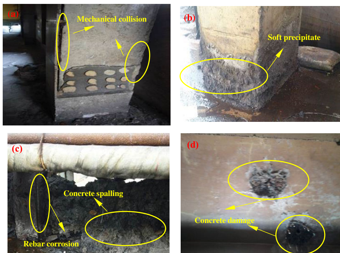
Figure 6. Appearance of concrete structure in the ammonium sulfate workshop. (a) The column in the warehouse; (b) the column in the synthesis section (outdoor); (c) the platform cornice in the vulcanization bed section; (d) the floor in the crystallization tank section.
