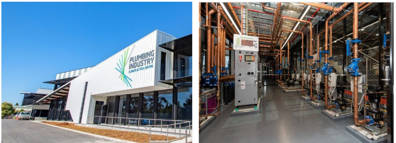
Figure 7. Case building and plant room.
