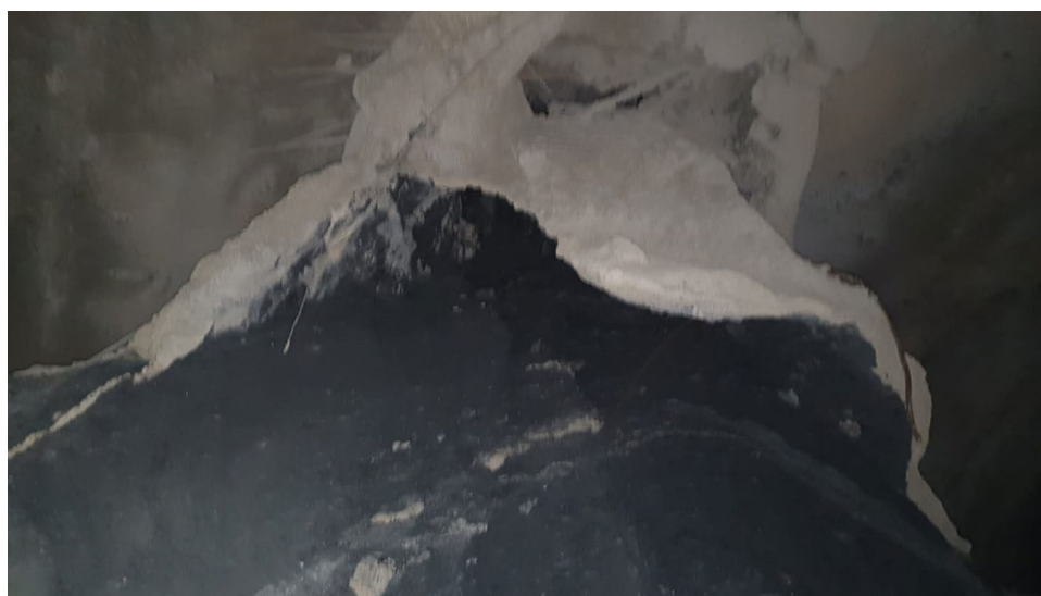
Figure 8. The tunnel collapsed section between km: 62 + 910 to 62 + 938.
