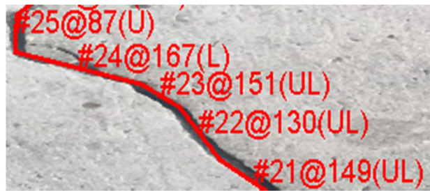
Figure 7. Example of a traced crack with the relevant information to be saved in a database.
