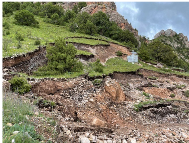
Figure 4. Tensile cracks in the trailing edge (2015.07).
