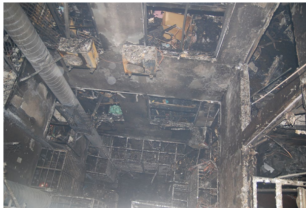
Figure 1. Burned situation in the atrium of the high-rise residential fire.
