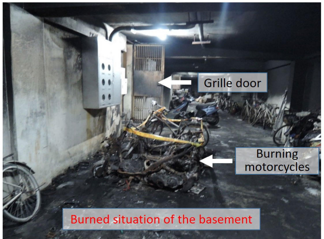
Figure 3. Description of the analyzed case (A) The appearance of the building. (B) The fire location in the basement.
