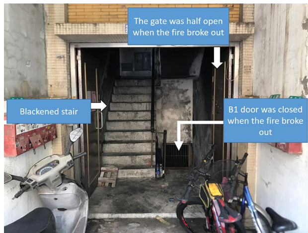
Figure 4. Blackened gate on the first floor.
