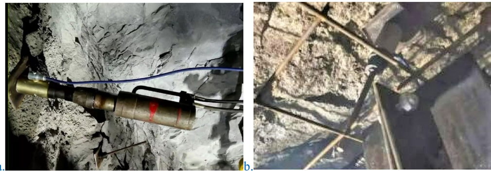
Figure 19. Real scene of the tensioning machine and the rock bolts. (a) Tensioning machine; (b) rock bolts.
