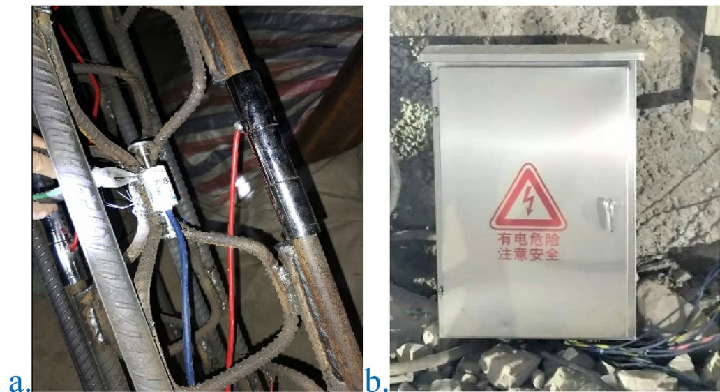
Figure 21. Actual view of the installation of the reinforcement meter and automatic monitoring instrument.
