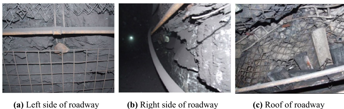
Figure 2. Deformation and failure of on-site roadway.
