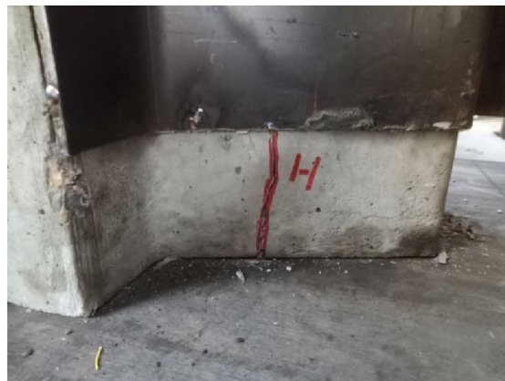
(a) Cracks at the bottom of specimens
