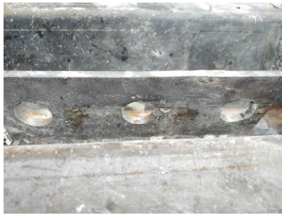
(a) Deformation of PZ shear connector
