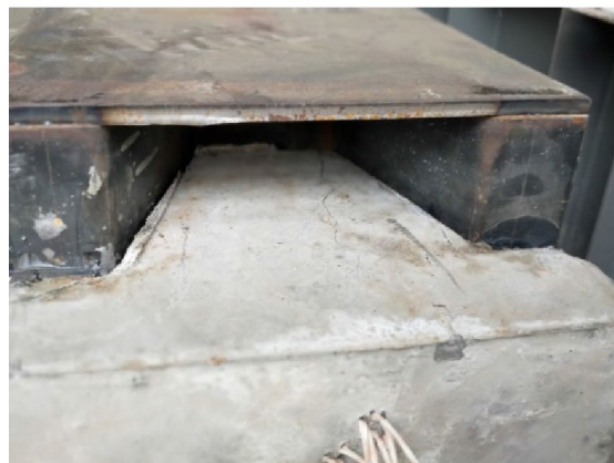
(b) Cracks at the top of specimens
