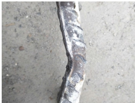
(b) Deformation of transversal reinforcement
