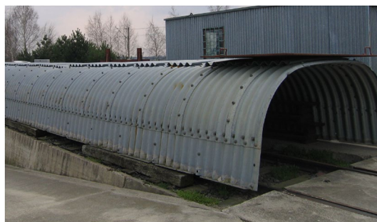
Figure 7. General view of the tested steel box structure.
