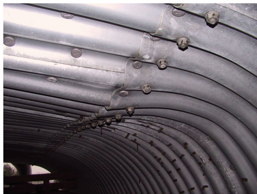
Figure 20. View of damage caused by concentrated load applied directly to the steel structure.
