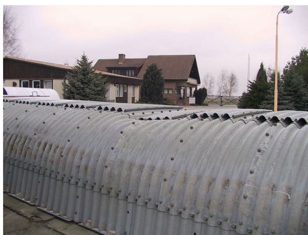
Figure 19. Local damage where the stiffness of the structure changes after the tests.
