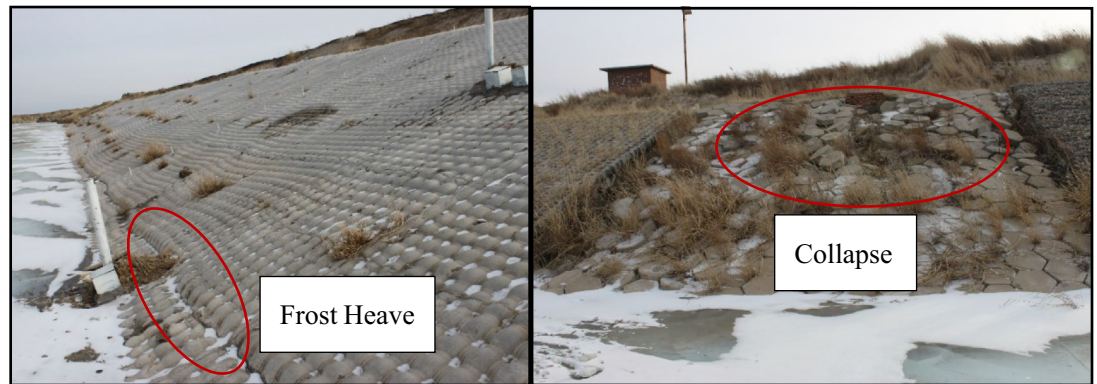
Figure 1. Frost damage to canals.
