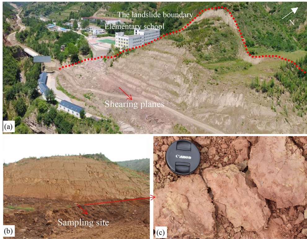
Figure 2. Sliding scratch surfaces and sampling site. (a) The landslide boundary; (b) sampling site; (c) sliding scratch surfaces.
