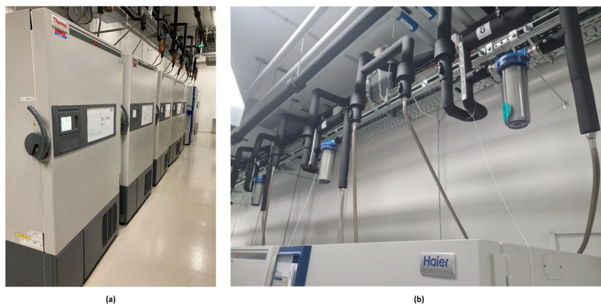
Fig. 1 (a) The room accommodating 53 ULT freezers. (b) The insulated chilled water pipes and multi-particle filters.
