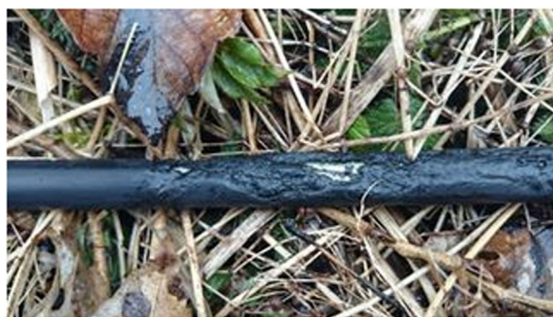
Fig. 7 Example of damaged insulation after prolonged contact with vegetation (tree).
