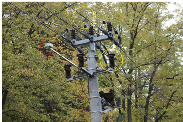
Fig. 10 Single pole with installed a galvanic contact method (yellow circles) and antenna based method (red circle).
