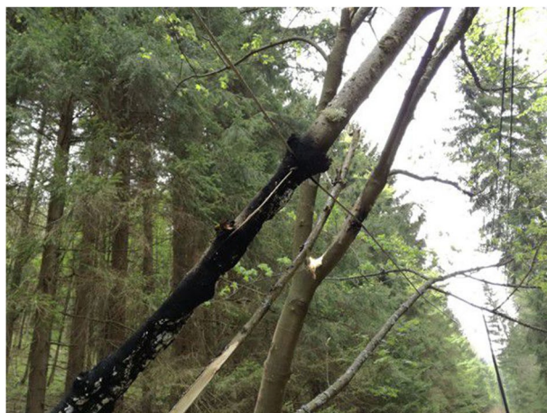
Fig. 11 Example of a burned tree after insulation failure.
