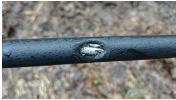
Fig. 8 Second example of damaged insulation after prolonged contact with vegetation (tree).
