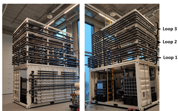
Fig. 1 Picture of the pilot plant of a drinking water distribution system (DWDS). The structure is 5.2 m × 2.6 m. The three identical loops are indicated.
