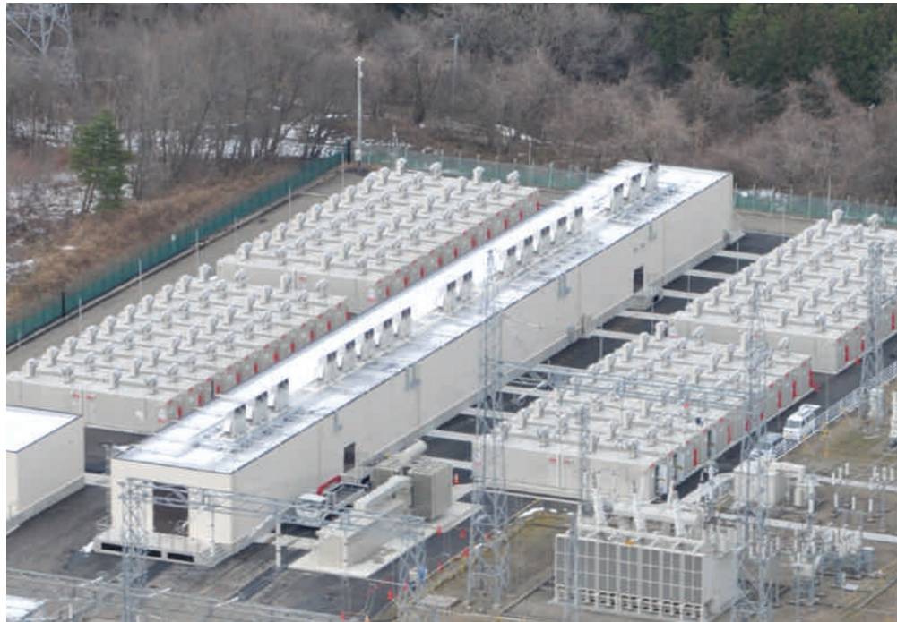
Toshiba has supplied Japan's Tohoku Electric Power Company with one of the world's largest lithium-ion battery energy storage systems.
