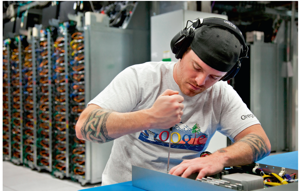
Figure 1. Zero-waste data centres. Google uses several circularity strategies at its globally owned and operated data centres, such as repairing components whenever possible to extend the life of servers.
