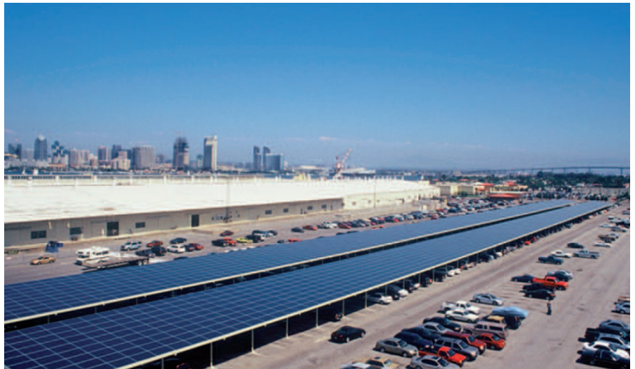
A 750-kilowatt solar-photovoltaic installation at a US Navy base in San Diego.
