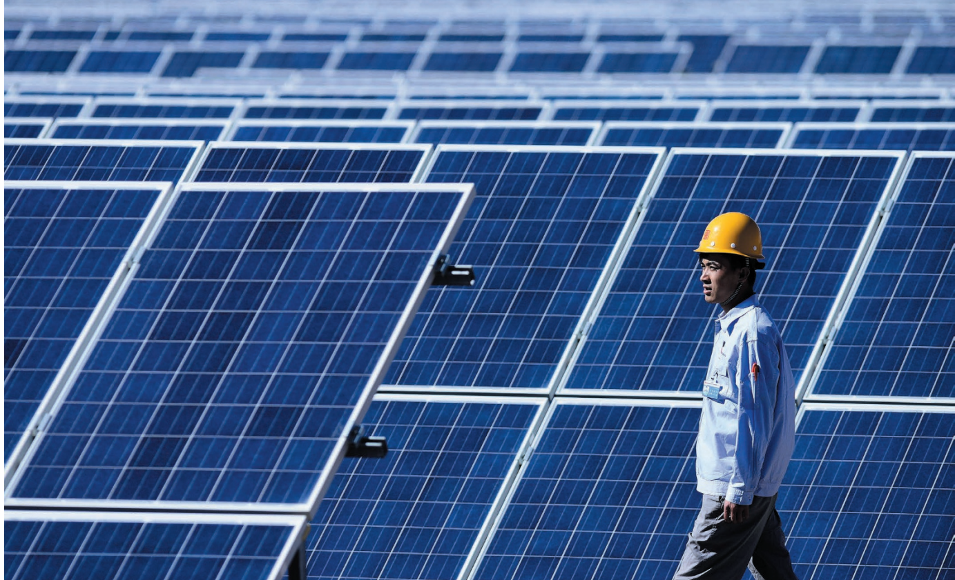
Solar panels in northwest China's Qinghai province.
