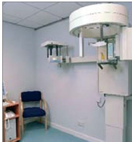
A typical x-ray room at OrthoWorld practices.
