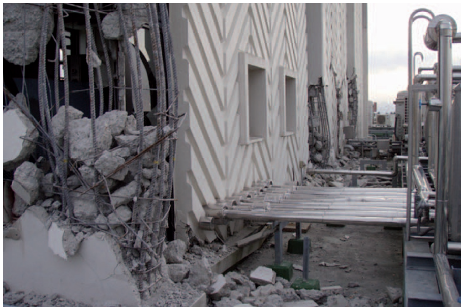
Some buildings at Tohoku University are too damaged to be entered safely.
