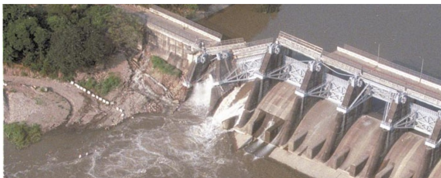
Dambuster: the Shihkang reservoir was damaged by the earthquake that struck Taiwan last week.
