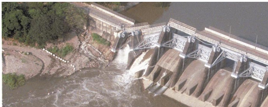
Dambuster: the Shihkang reservoir was damaged by the earthquake that struck Taiwan last week.
