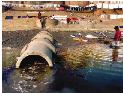
Pipe dream: India plans to harness rivers such as the Ganges to improve access to clean water.
