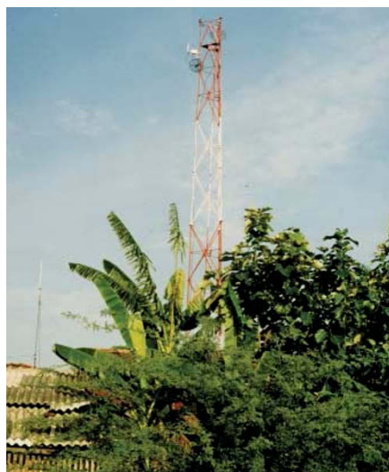
Touching base: transmitters connect corDECT users up to 25 kilometres away to the central unit.
