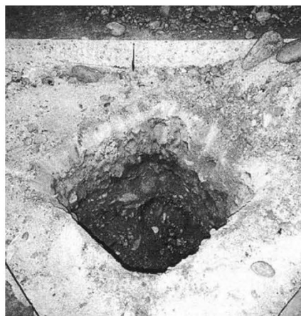
The alluvial terrain appears below the compacted grave, sand and concrete beneath the floor of the ESRF; a pen indicates the thickness of the slab.
