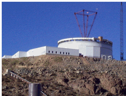
Going up: the Gemini facility at Cerro Pachon, Chile, pictured last month.
