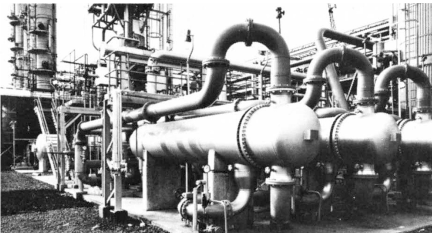
Heat exchangers at VCM plant
